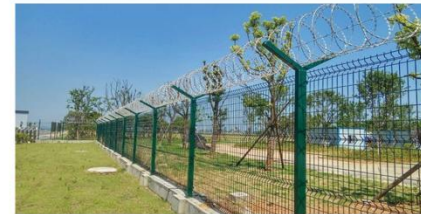
Welded Mesh Fence
